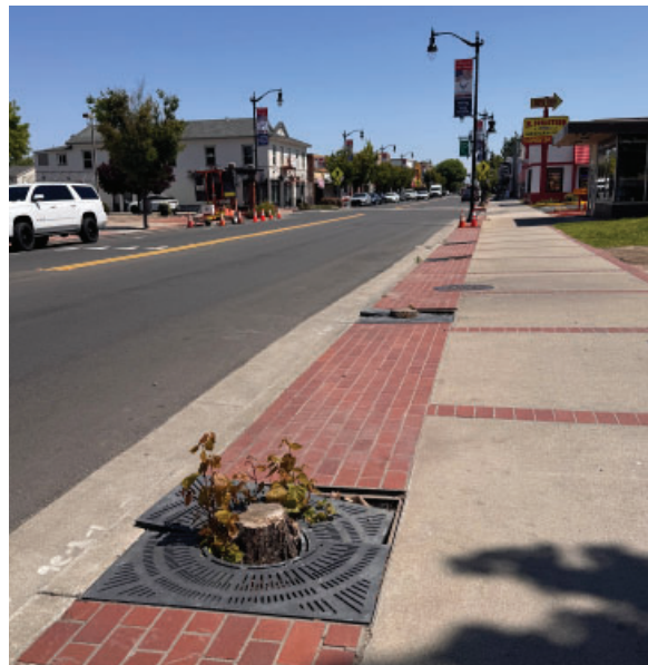
Failed tree planting at a tree planter on W. Yosemite Ave with tree grates and brick paving.
